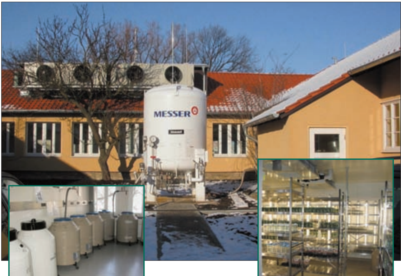
Fig. 15: The new facilities of the working group in the Vavilov House of the IPK renovated in the year 2004: An integrated supply system provides the nitrogen from a central (middle picture) to the storage tanks (left) containing a total storage capacity of 65,000 tubes. In vitro slow growth storage is performed in two cold and two warm culture rooms comprising 110 m 2 of storage area in illuminated shelves (right) (J. Keller).
